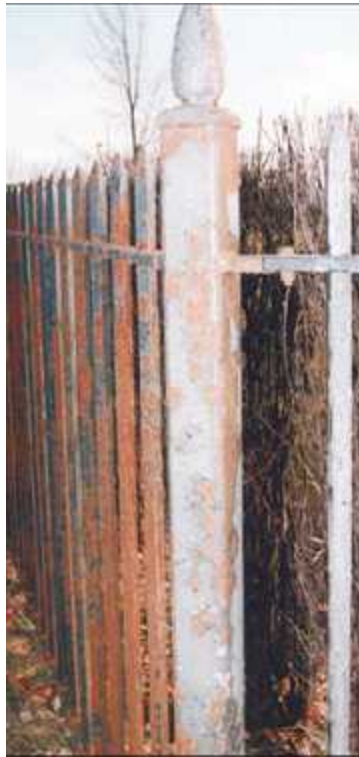
This steel fence, which is set back from a main thoroughfare about 20 feet, illustrates the corrosive effects of road salt used in northern communities to melt ice and snow.
